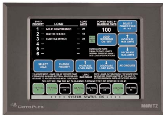
Advanced electronic power control : Octoplex (above) can even manage load shedding on a yacht with two shore power cables.
